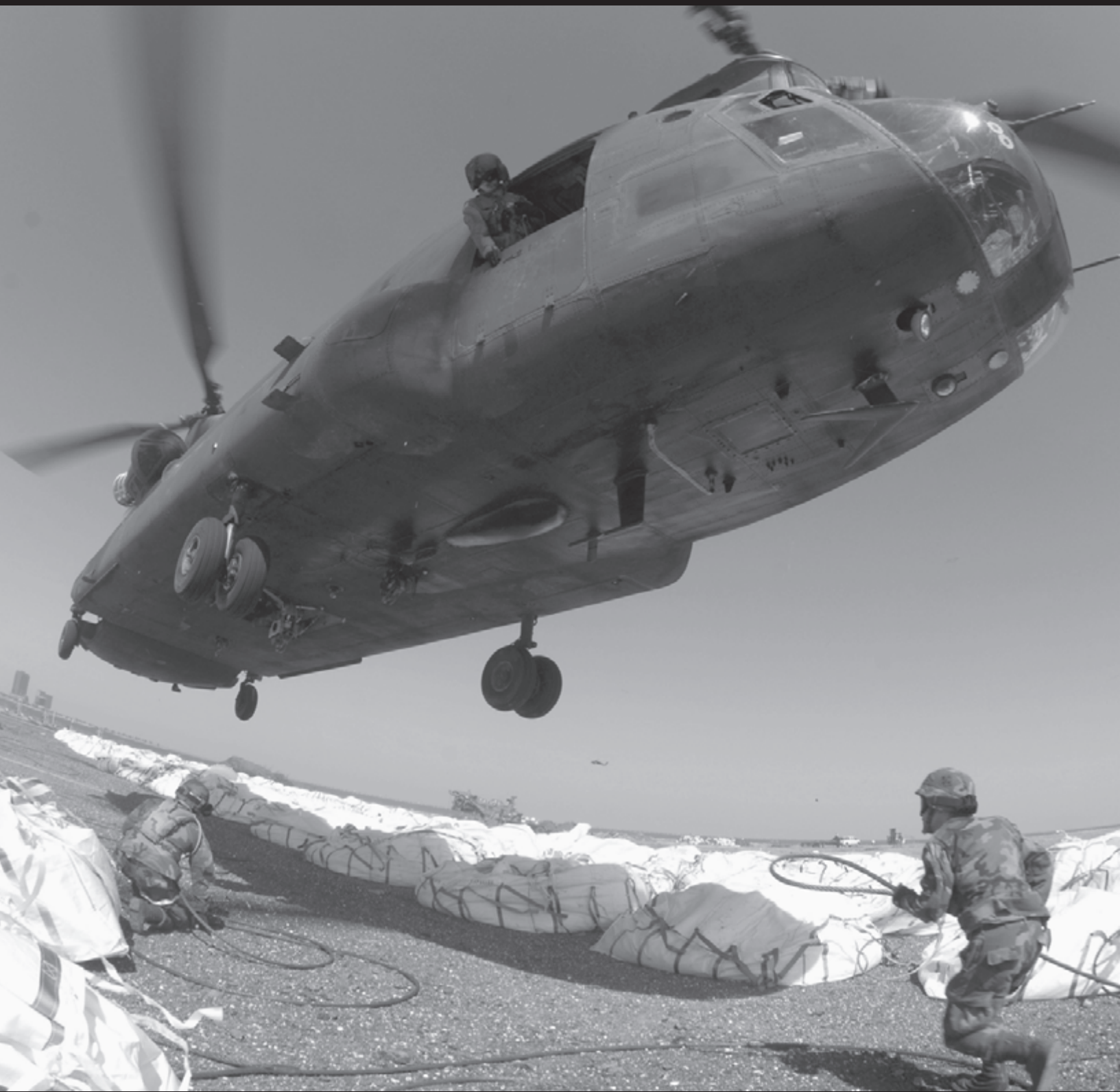
Army National Guardsmen Spc. Clint Aucoia from Morgan City, La., and Pfc. Christopher Tiffit from Spokane, Wash., attach hooks supporting large bags of sand to a CH-47 Chinook helicopter in New Orleans, La., on Sept. 7, 2005. The bags are being used to plug the levee that burst during Hurricane Katrina. (DoD Photo)
